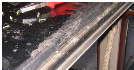
Deterioration was worst at the rear of the roof
