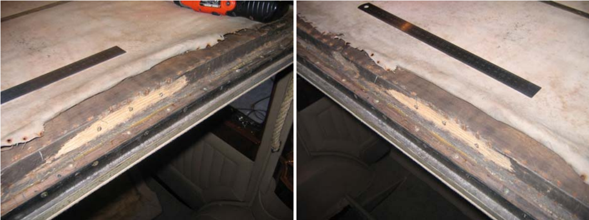
Water had taken it's toll on the woodwork at the back of the roof.
